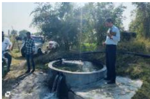
Photo 18: Pipeline for irrigation
